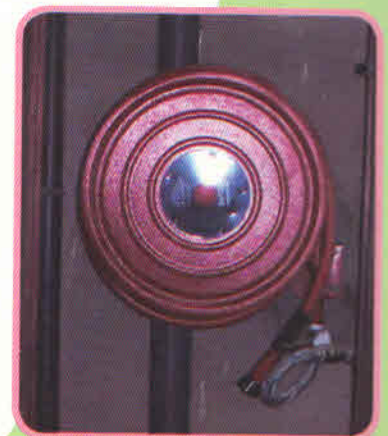
Fire hose station
